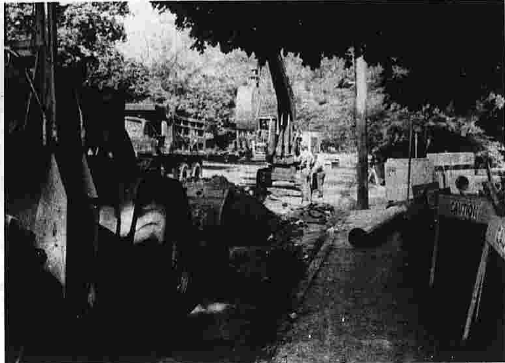
Work is progressing along Porter Street on a project designed to drain surplus water from a pond at Porter Street and Adelaide Road and prevent it from flooding houses on Richard Road. (Herald photo by Pinto)
